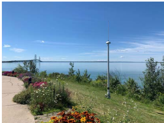
New freshwater HF Radar installation at the confluence of Lakes Michigan and Huron. Credit: Brian Zelenke, NOAA.
