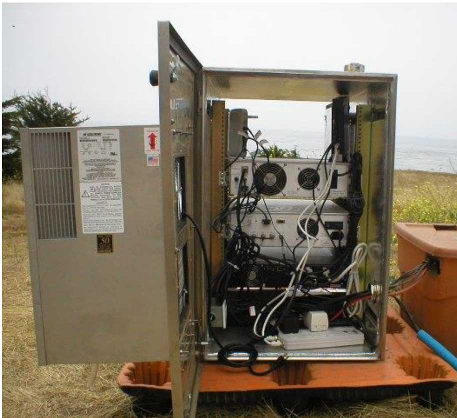
Figure 2. View of outdoor electronics enclosure with both doors open. Air conditioner is attached and all HFR electronics are mounted within the enclosure.
